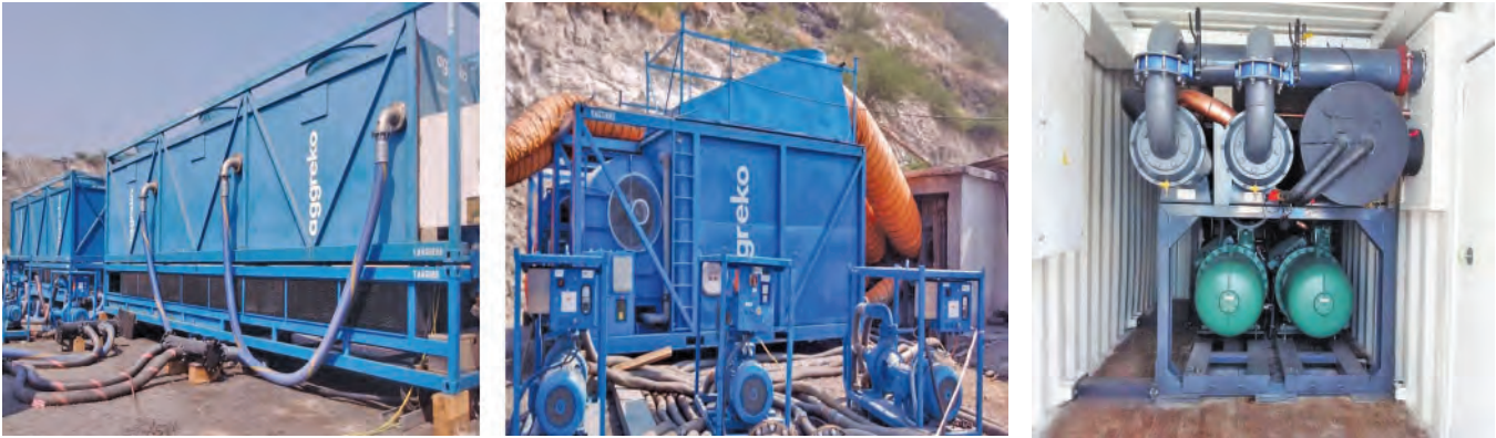
Fig.3 (a) and (b) Cooling tower and bulk air handling unit
