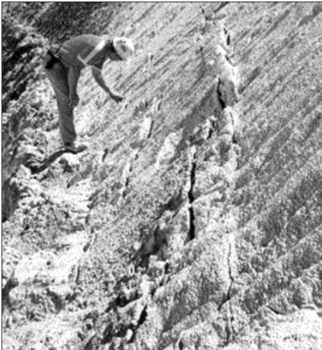
Fig.12: Slumping of weak rock at the bottom of an open pit. The cracks show local failures have occurred in the area and can spread (not own and not of the mine, Courtesy: Szwedzicki T. (2003) ).
