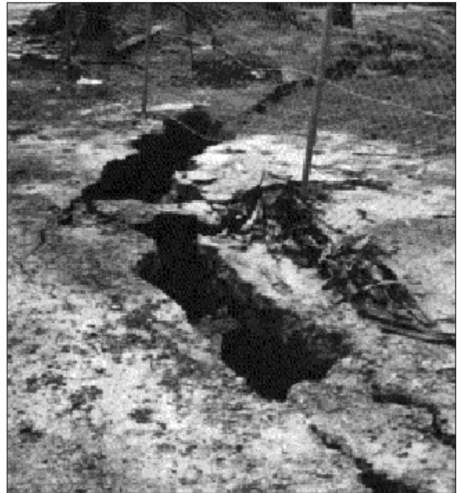
Fig.13: Progressive opening of cracks at a periphery of an open pit. If the cracking spreads even after filling, the signs are dangerous and must be monitored (not own and not of the mine, Courtesy: Szwedzicki T. (2003) ).
