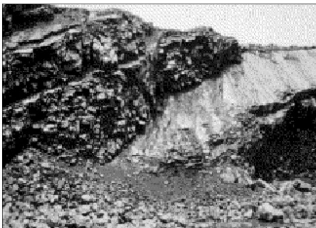
Fig.11: A slicken sided plane facilitating failure of a slope. In the interfaces of weak and jointed rocks with soil in contact with a massive block of rock with sharp surfaces, the failure can take place along the sharp surface, when wet (library picture, not own and not of the mine, Courtesy: Szwedzicki T. (2003) ).
