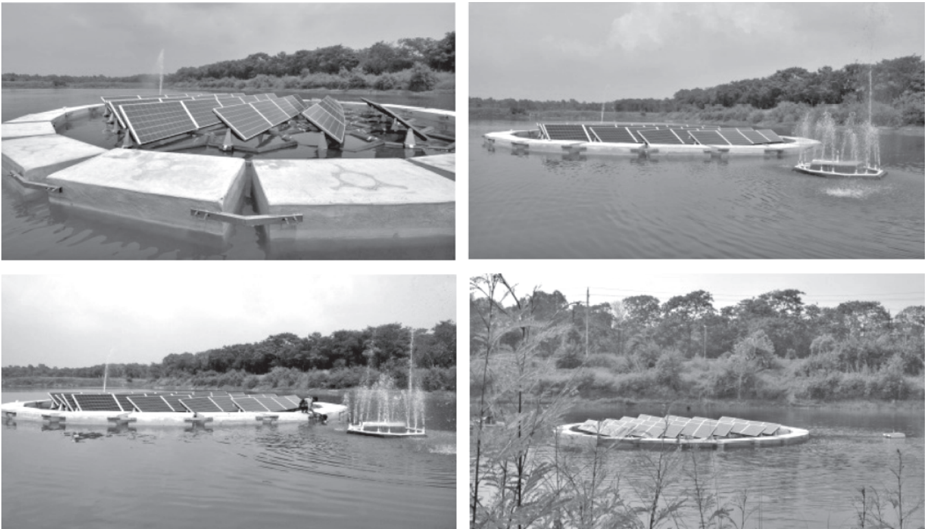
Fig.6 10 kW floating solar plant with dual axis tracking capabilities at Dhanas Lake, Chandigarh installed by Yellow Tropus Pvt Ltd
