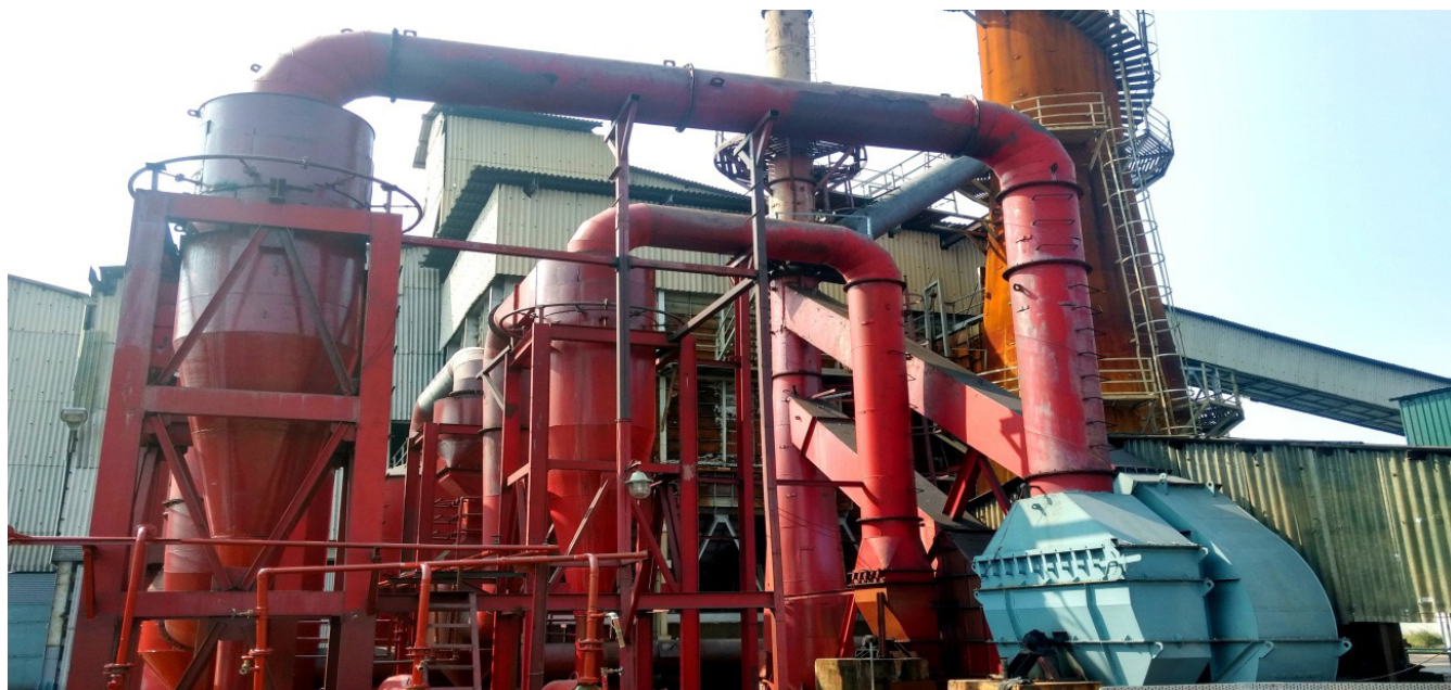
Figure 1. The Venturi scrubber setup.
