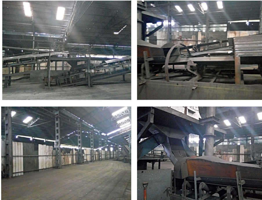
Figure 5. Open transfer points, open/temporarily covered belt conveyor, floor-laden dust and roof ventilating leakages as found during the visit.
